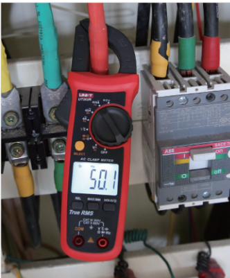
High voltage (600V) frequency measurement
